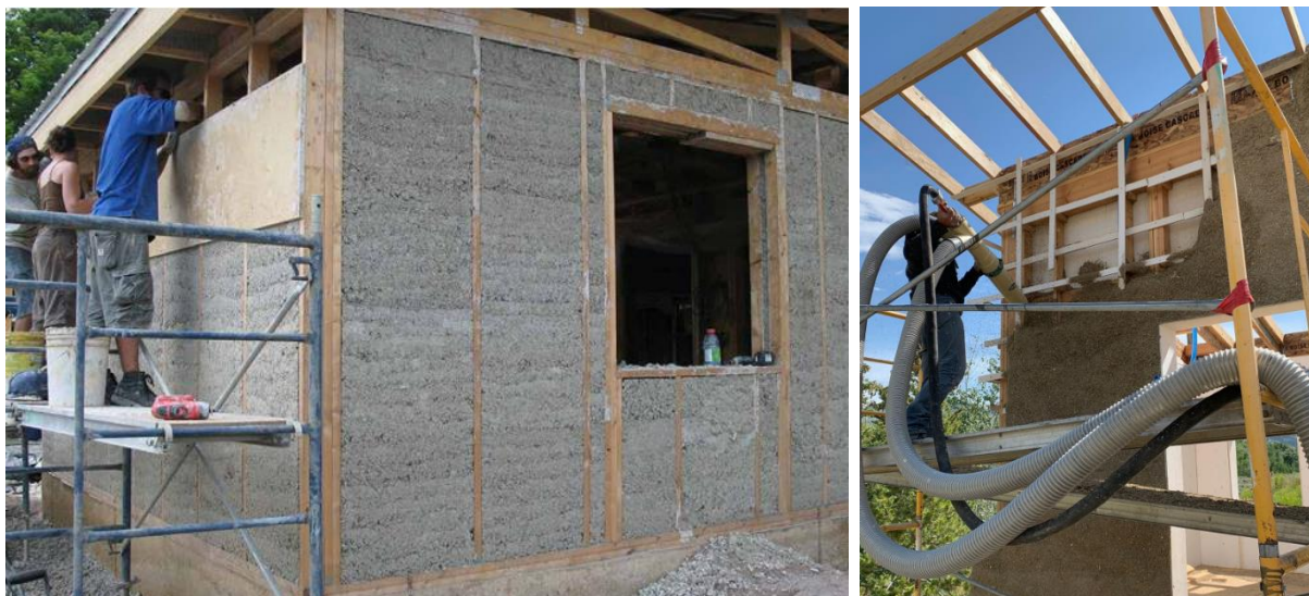
Figure. 1. Using hemp concrete by mixing at a construction site for the construction of wall structures
